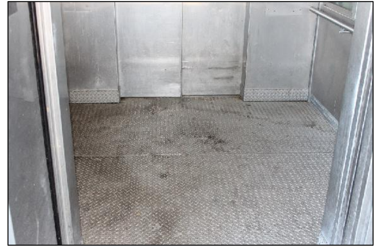
Unsanitary elevator conditions contribute to an unpleasant transferring experience.
