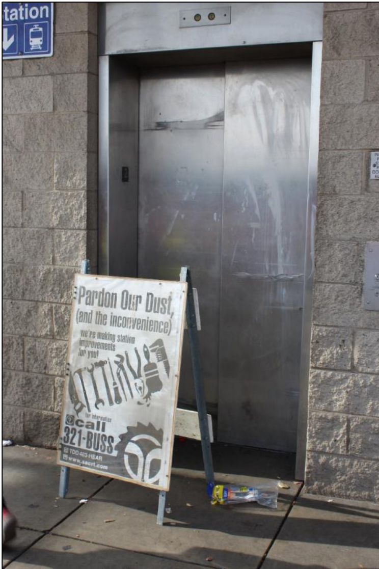
Fixing and replacing the elevators is a major priority for riders.
