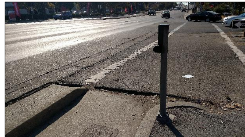
Freeway off-ramp crossings have narrow ramps and poor pavement conditions.
