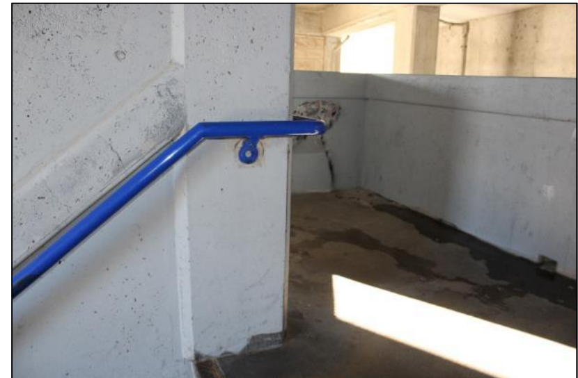
Sharp corners block visibility on the stairs.
