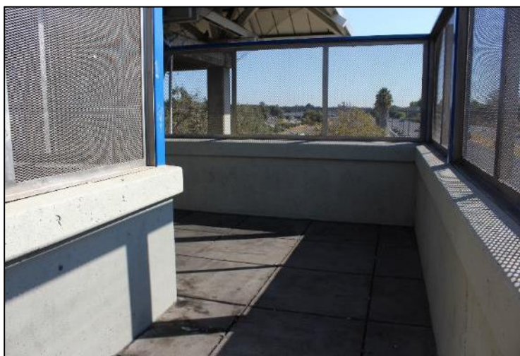
Sharp corners hide the stair access point. Concrete and shade structures create dark areas and prevent natural light from entering the space.
