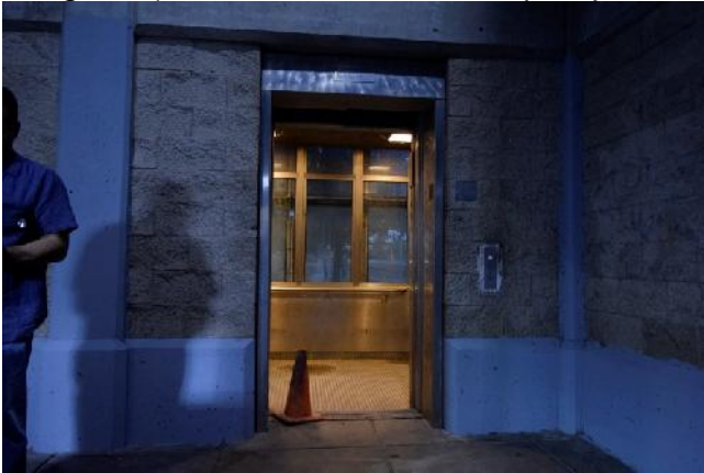
Image 21 (elevator door stuck in open position. Note puddle of unknown liquid on floor)
